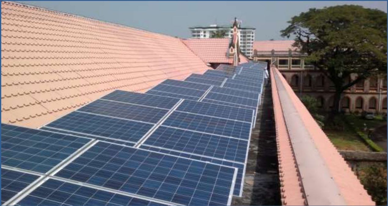
30kWp Grid connected Solar Power Plant at St Joseph Pontifical Seminary, Ernakulam
